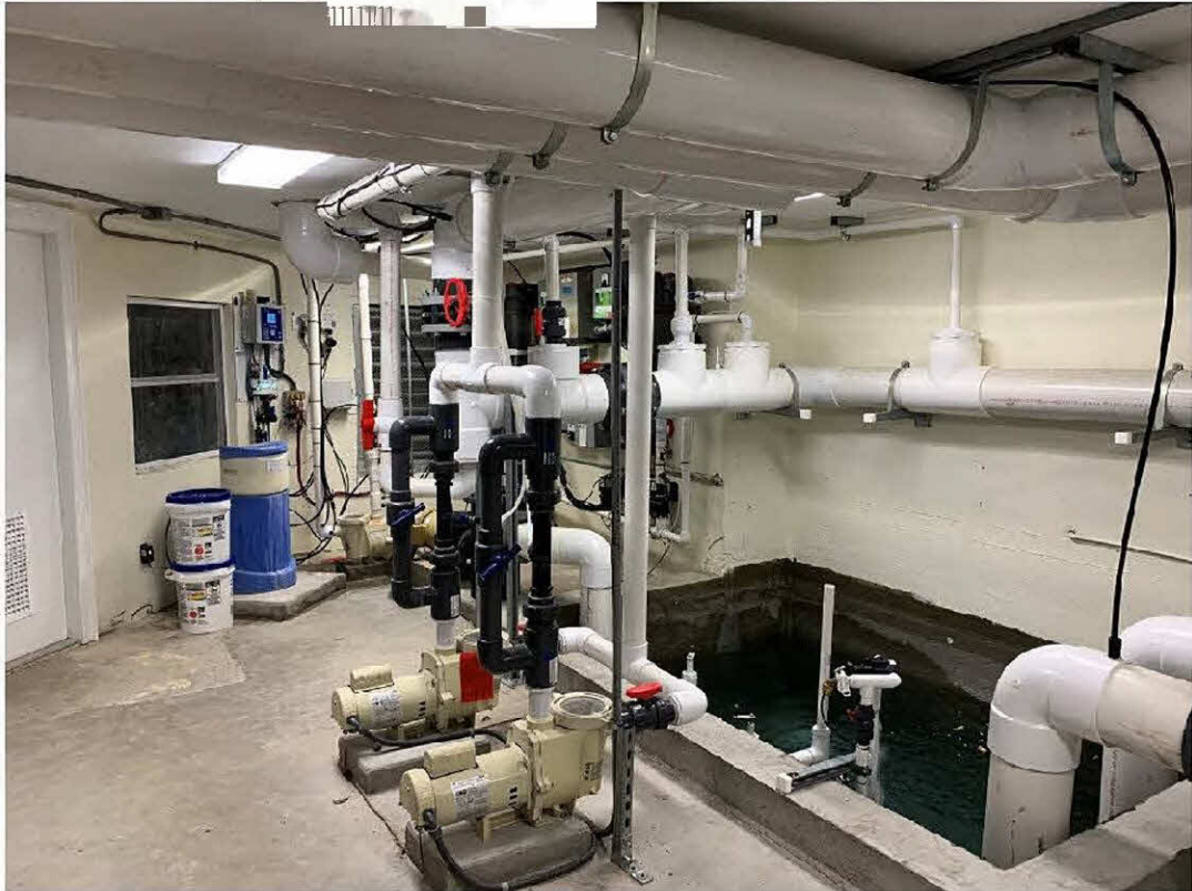
New Control Pump Room
