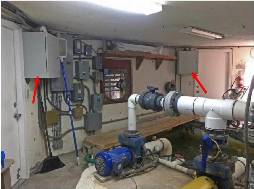
Old Pump Control Room
